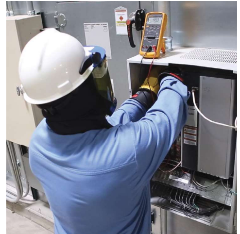
Figure 1. Absence of voltage test using a hand-held voltage test instrument.
